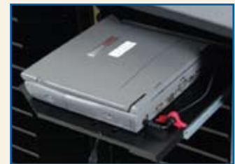
Wire management also located in tray on student side
